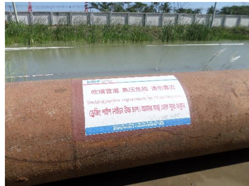
Safety caution in the dredging pipeline
