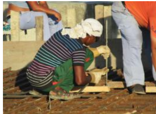
Without Safety Boot (NEPC workers)
