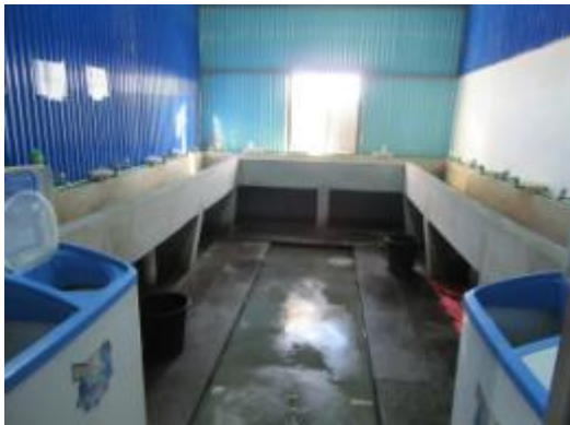
NEPC Workers Shower and Laundry Facilities
