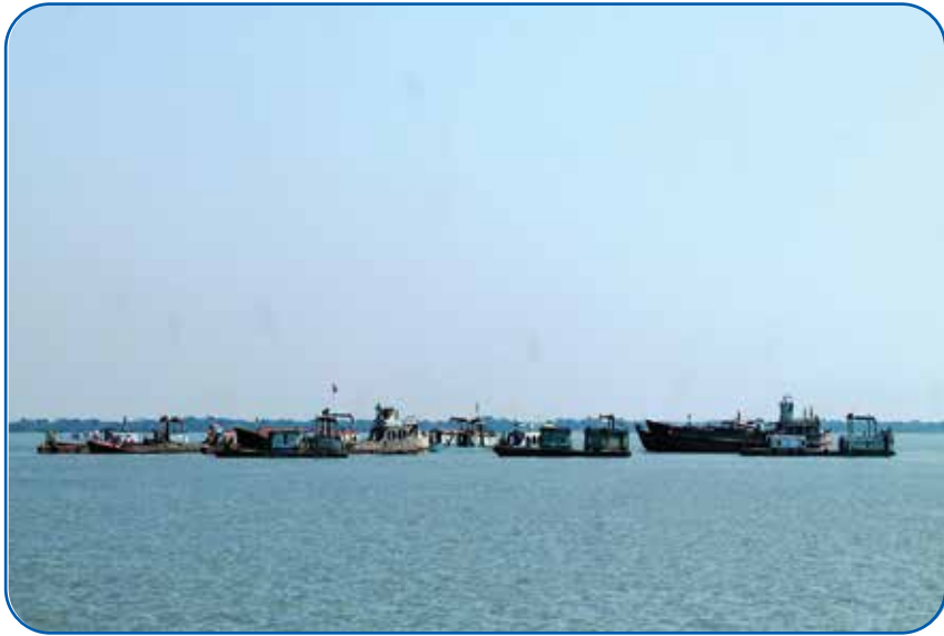
Loading Dredger with Sand for the Land Development of Payra 1320 MW TPP Project
