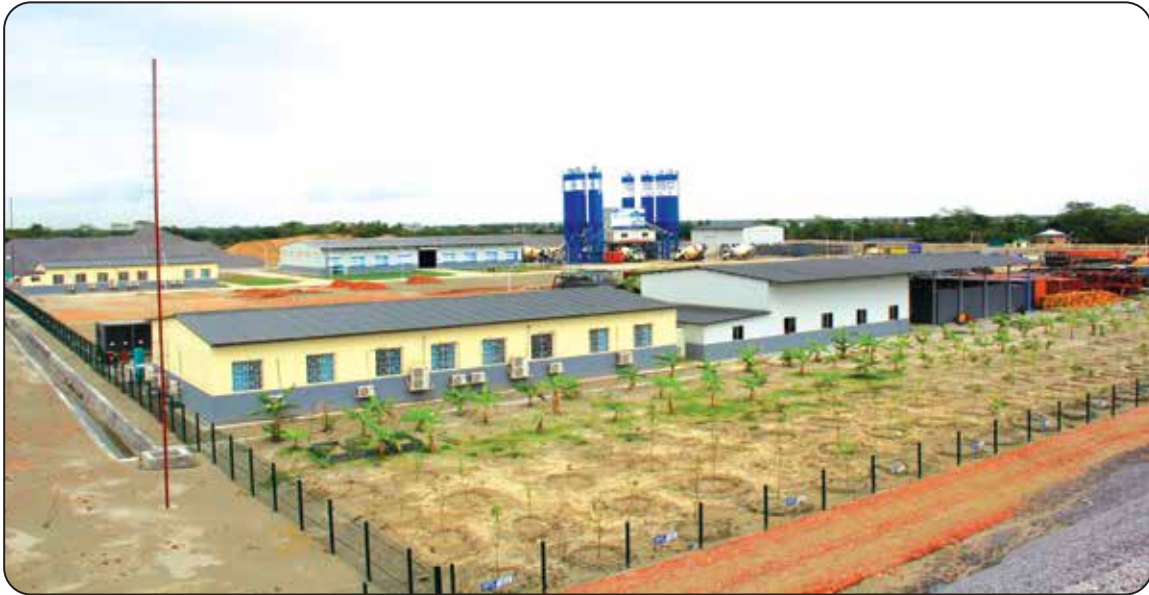
Concrete Batching Plant Area at Payra 1320 MW Thermal Power Plant Project Site
