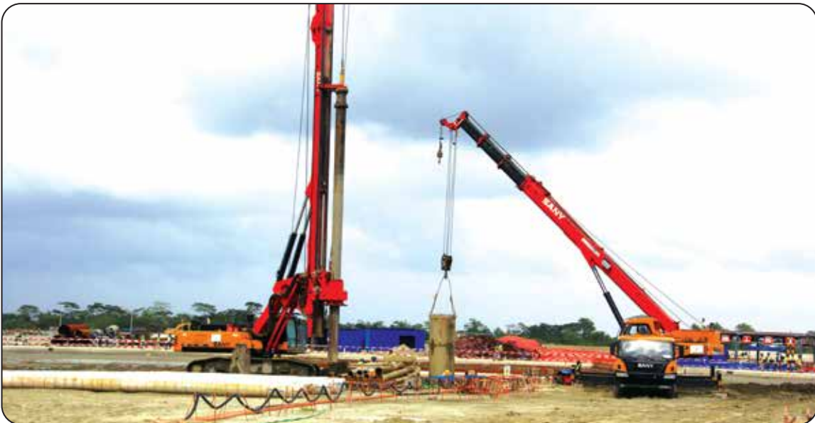
Service Pile in the Coal Yard for Payra 1320 MW Thermal Power Plant
