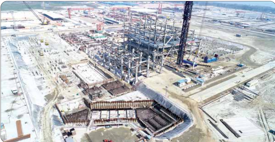
Overall Power Block Area for Payra 1320 MW Thermal Power Plant
